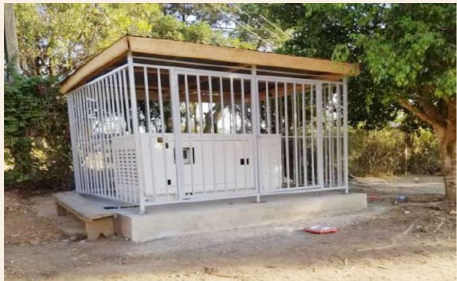
The newly procured generator for Mubende High Court
