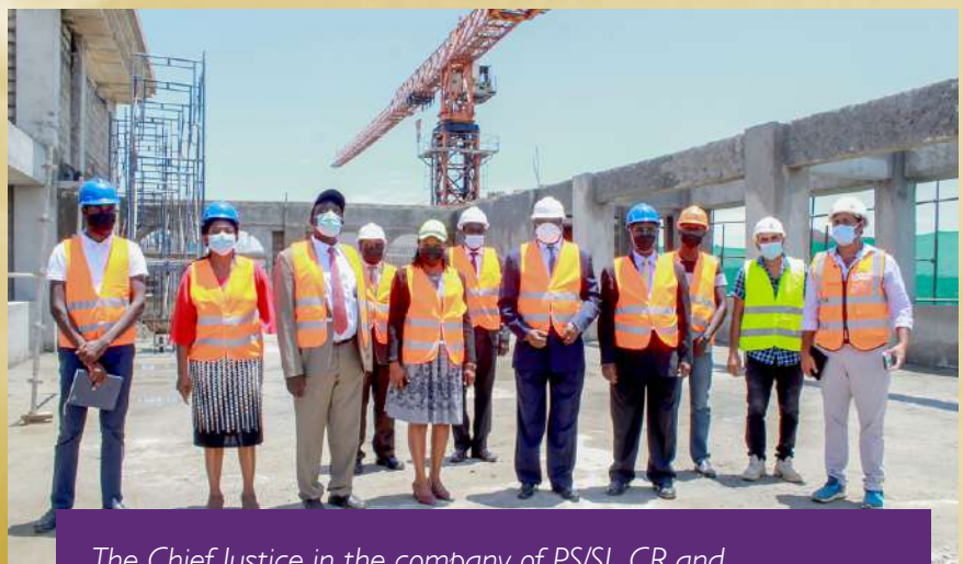
The Chief Justice in the company of PS/SJ, CR and Commissioner Engineering & Technical Services inspecting the Supreme Court and Court of Appeal construction premises
