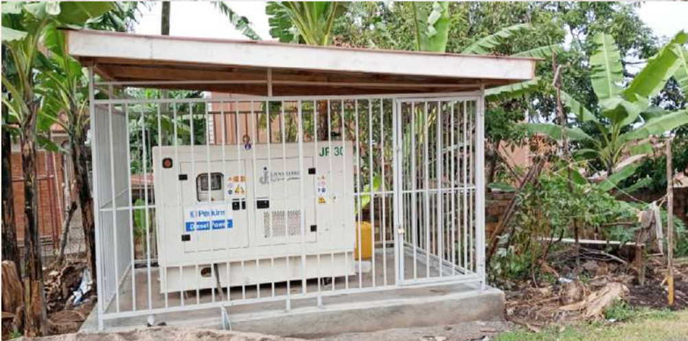
The new generator installed and tested at the Rukungiri Chief Magistrates Court
